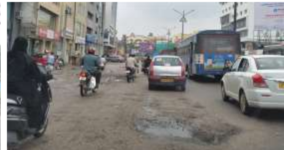
Pothole + Muddy Road
